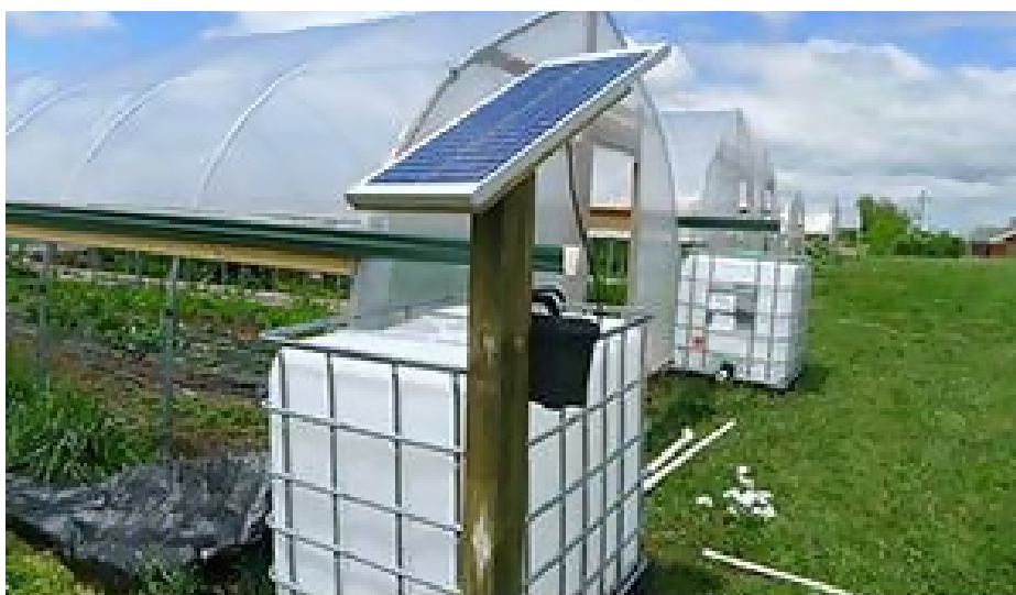
Rainwater catchment and solar + gravity-fed drip irrigation system being installed for flower crops in a high tunnel at Greenhouse 17
